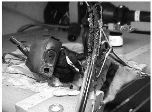
Fig. 12. Battery pack explosion after overcharging.
